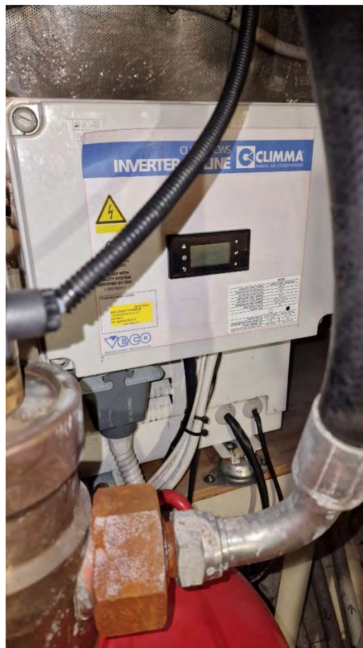
Photo 58 Air conditioning system.
