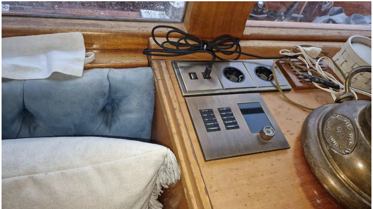
Photo 28 TV control system for the salon area.
