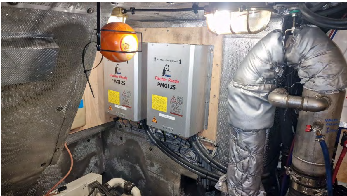
Photo 54 Main engine's exhaust and electronic control units of diesel generators.
