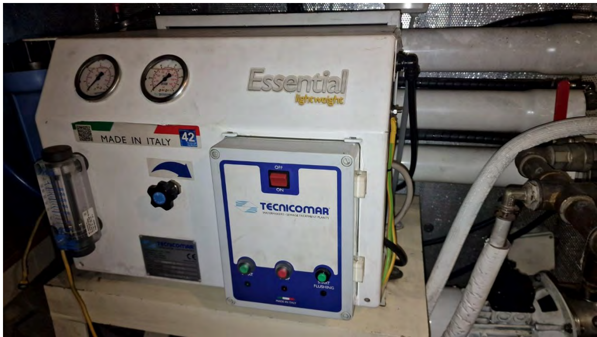
Photo 57 Water making system.
