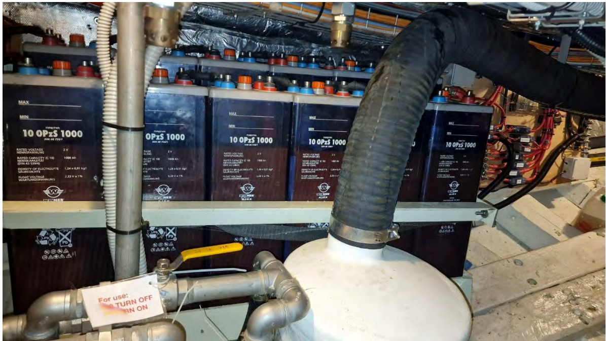
Photo 56 Set of batteries.
