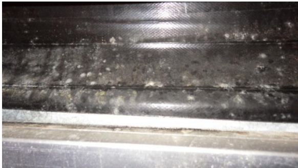
WHITE MOLD IN GALLEY
