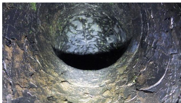
STARBOARD ABOVE WATER M/E EXHAUST
