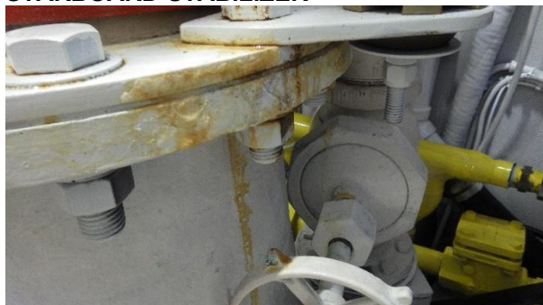
WATER LEAK PORT M/E EXHAUST
