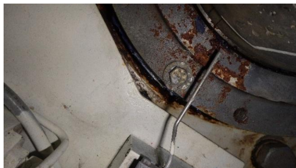
WATER LEAKING FROM PORT FIN
