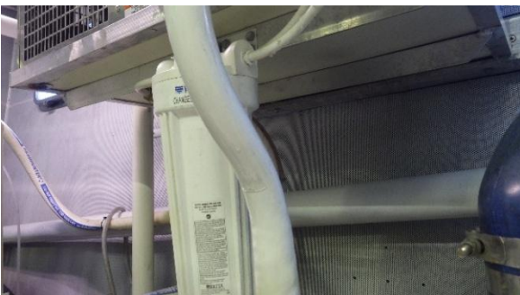
WATER LEAKING FROM DISPENSER
