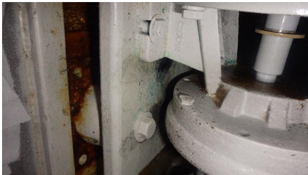
CORRODED FEET ON CHILL WATER PUMP
