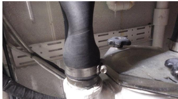
RAW WATER SUCTION HOSE COLAPSED
