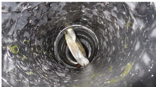
PORT ABOVE WATER M/E EXHAUST
