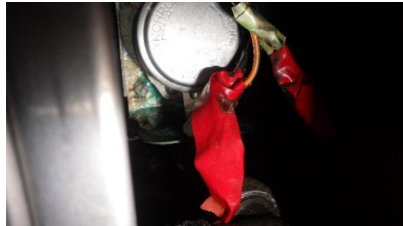
RESIDENTIAL WIRE JOINTS ON WIRING
