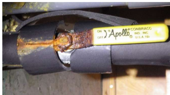
HEAVY CORROSION ON ISOLATION VALVES AT EACH FAN COIL UNIT
