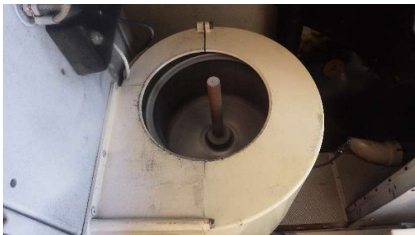
PROTECTIVE GRILL MISSING FROM SQUIRREL CAGE BLOWER ABOVE CHILLERS
