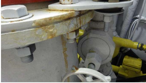
WATER LEAK PORT M/E EXHAUST
