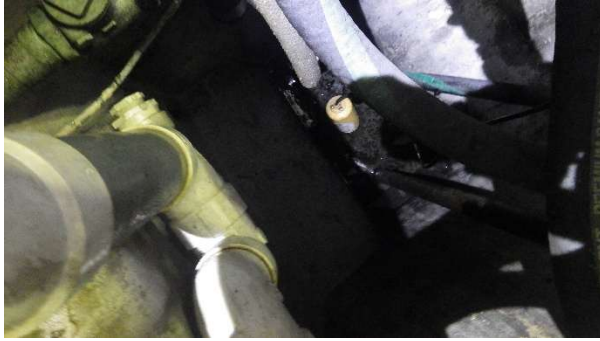
NEOPRENE INSULATION FAILING THROUGHOUT THE VESSEL. MULTIPLE OVERHEAD LEAKS NOTICED.
