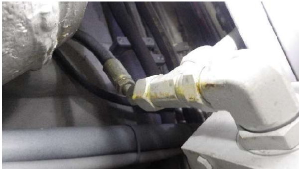
HYDRAULIC OIL LEAKING STARBOARD STABILIZER
