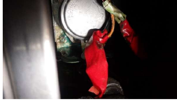
RESIDENTIAL WIRE JOINTS ON WIRING
