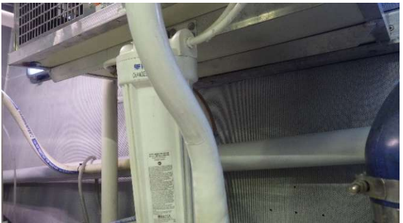
WATER LEAKING FROM DISPENSER
