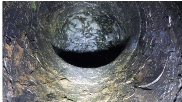
STARBOARD ABOVE WATER M/E EXHAUST
