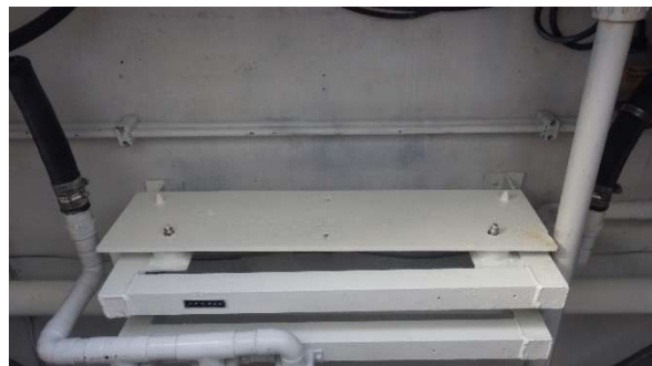
MISSING BILGE PUMP MOTOR ASSEMBLY IN LAZARETTE
