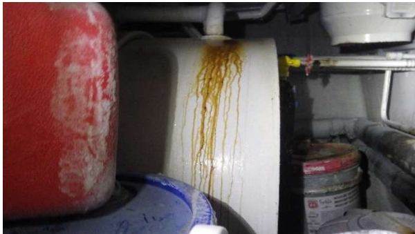
CONDENSATE FREELY DRIPPING INTO BILGE UNDER CHILLER RACK
