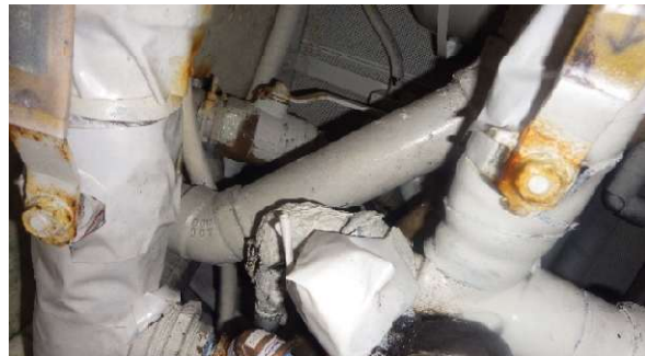
SEIZED VALVES UNDER HVAC CHILLER
