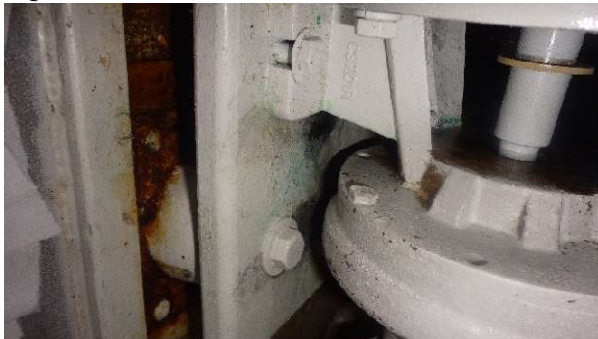
CORRODED FEET ON CHILL WATER PUMP
