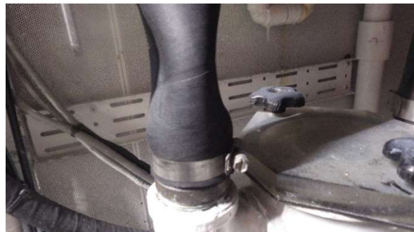
RAW WATER SUCTION HOSE COLAPSED
