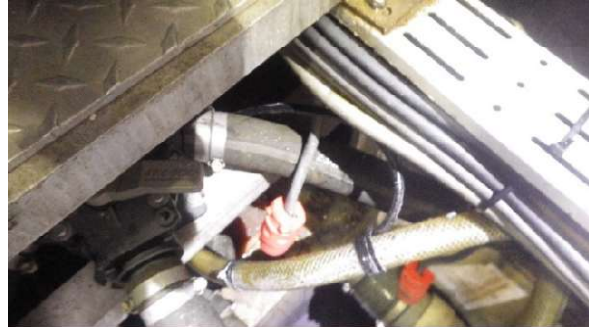
LOOSE 120VAC OUTLETS HANGING OUT CENTERLINE BILGE ENGINE ROOM
