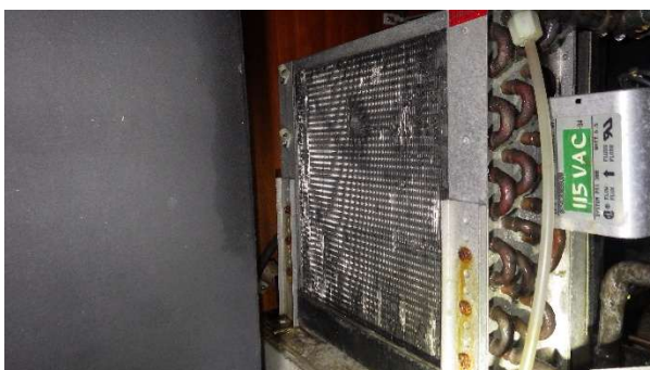
NO AIR INTAKE SCREEN ON MISC. FCU'S
