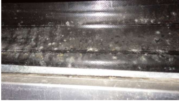
WHITE MOLD IN GALLEY
