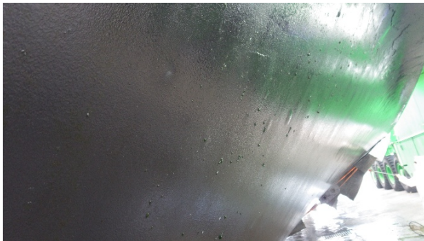
HUNDREDS OF BLISTERS UNDER THE BOTTOM PAINT MOST LIKELY DUE TO PAINT APPLICATION FAILURE. DOES NOT LOOK OSMOTIC
