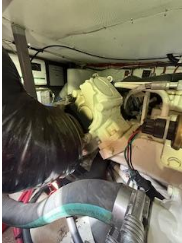
The port engine has an exhaust leak at the turbo outlet flange.
