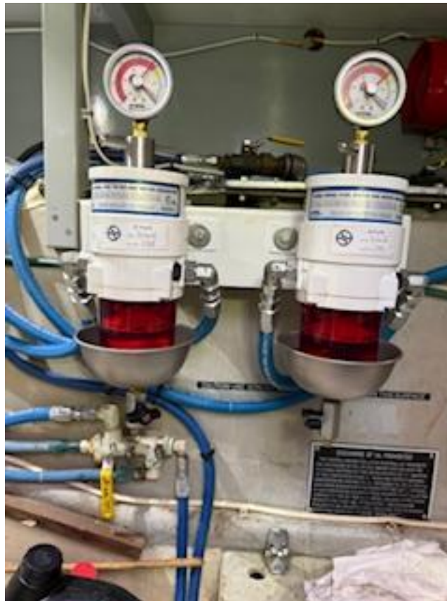
Both main engines are equipped with a single Racor fuel/water separator Model 500MA.
