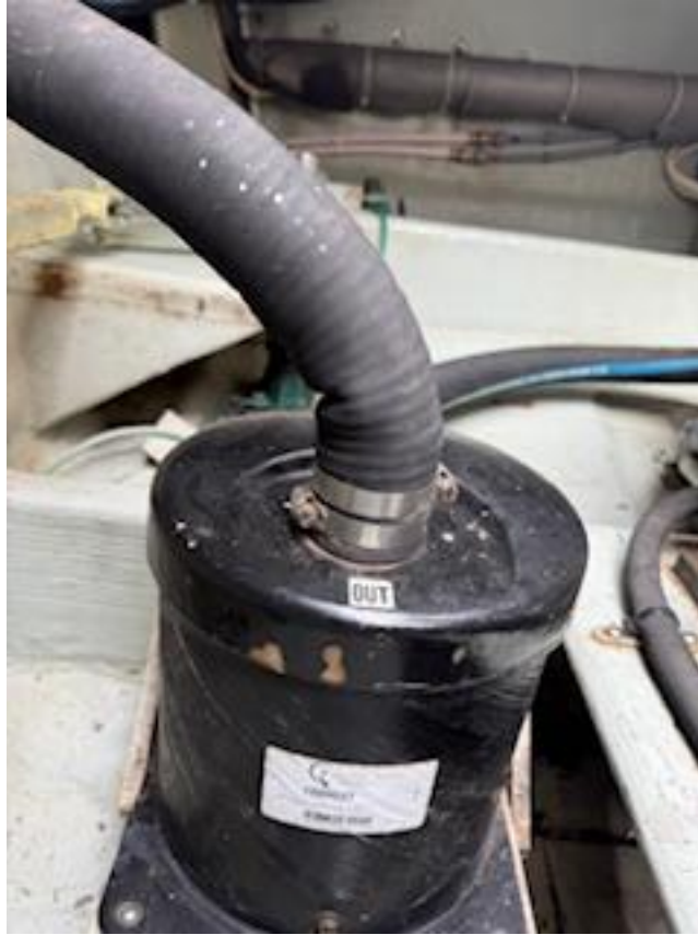
The generator muffler outlet hose is partly kinked.
