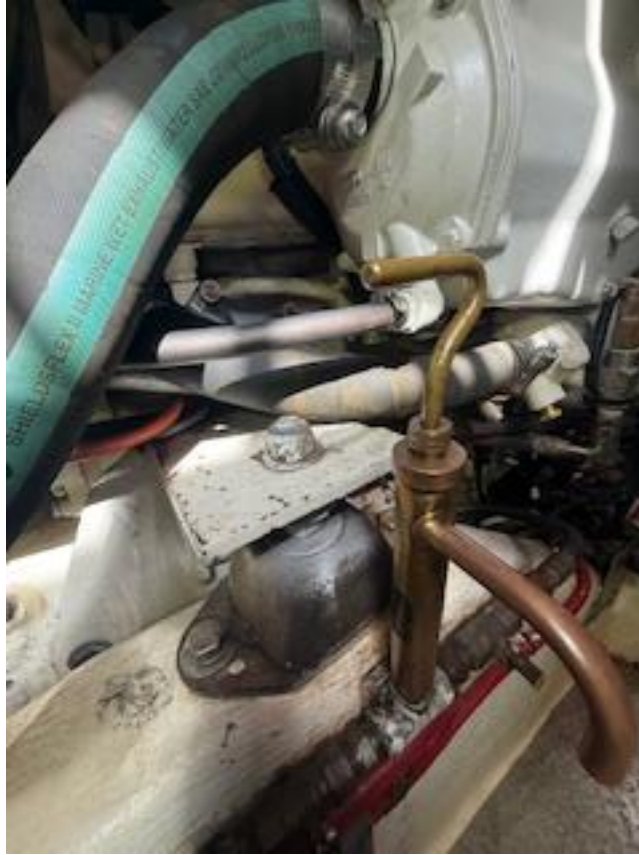
The port engine has a sea water hose chaffing on the right rear engine mount.
