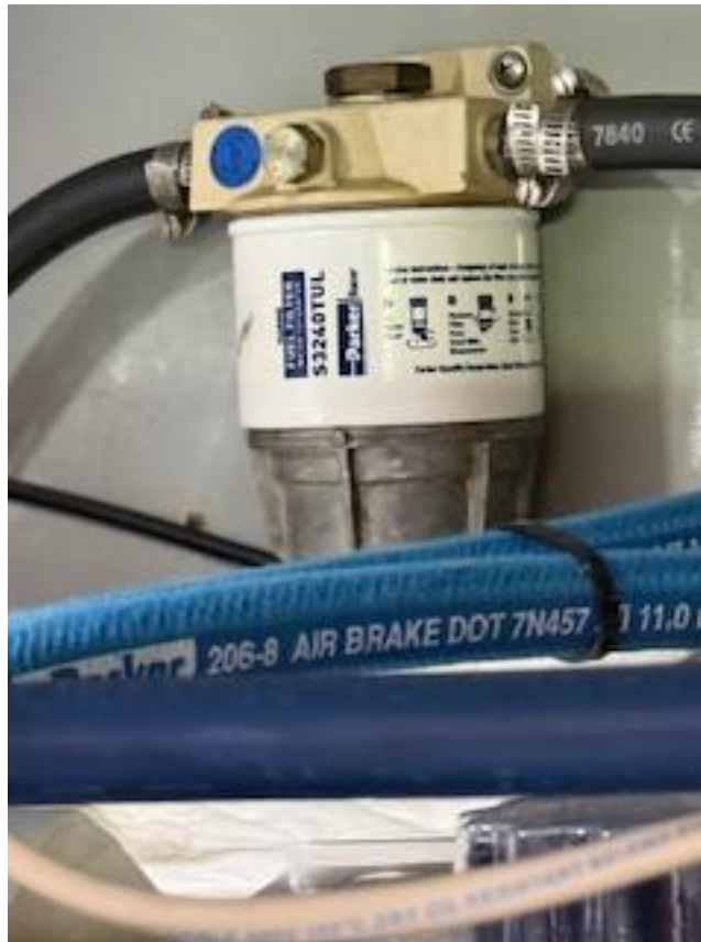
The generator is equipped with a single Parker/Racor fuel water separator. Part number S3240TUL.
