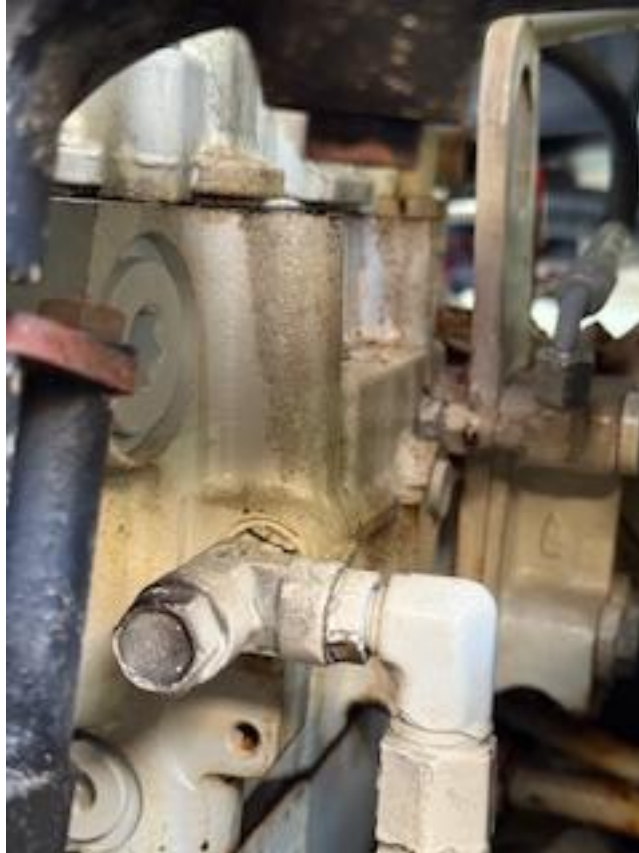
There is a small oil leak coming from the starboard engines' lower valve cover gasket.
