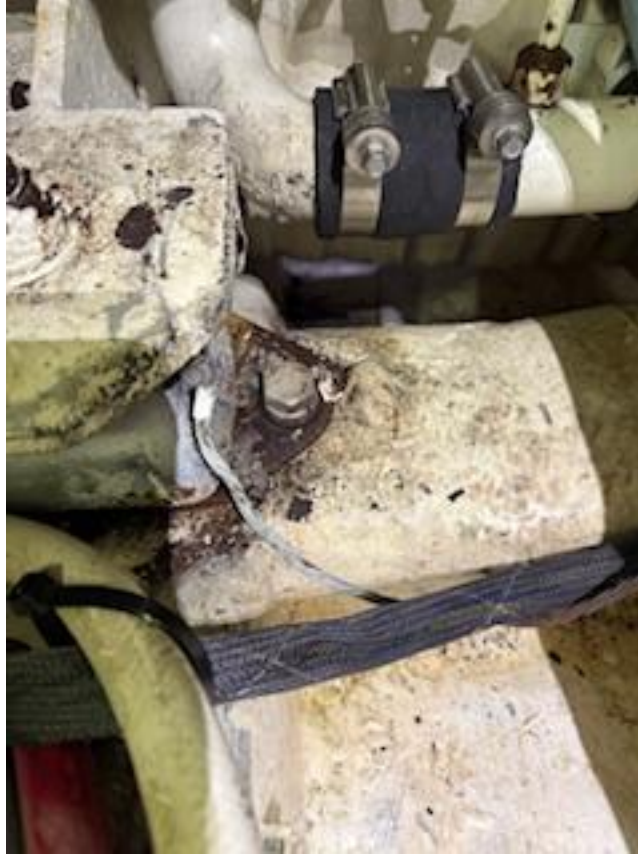
The port engine left front has a broken grounding wire by the left front engine mount.
