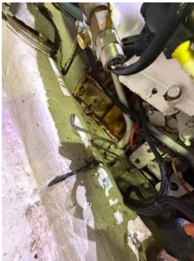
The starboard engine also has a broken grounding wire by the right front mount.
