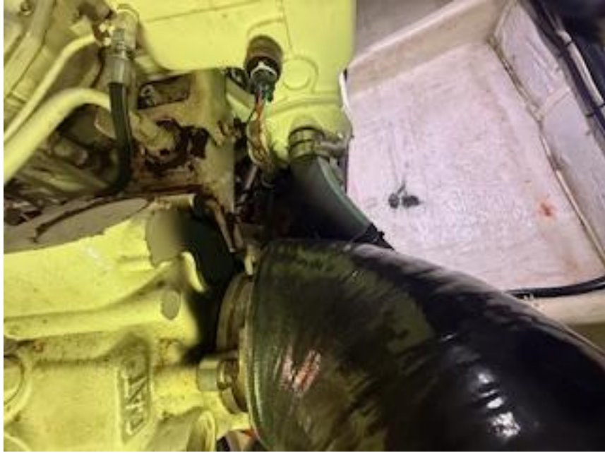
The starboard engine also has an exhaust leak at the turbo outlet flange.
