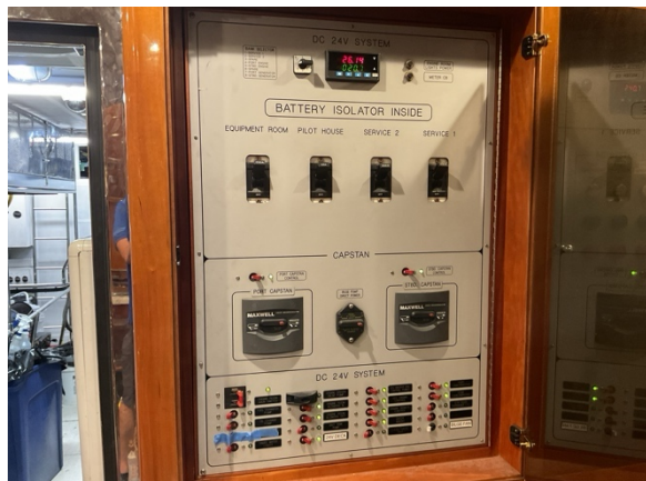
Electrical panel in ECR
