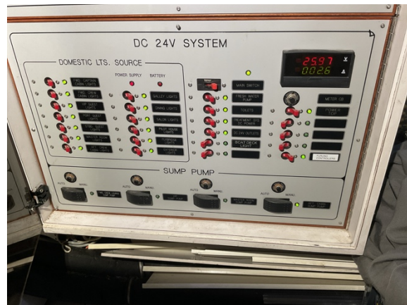
Electrical panel in doghouse
