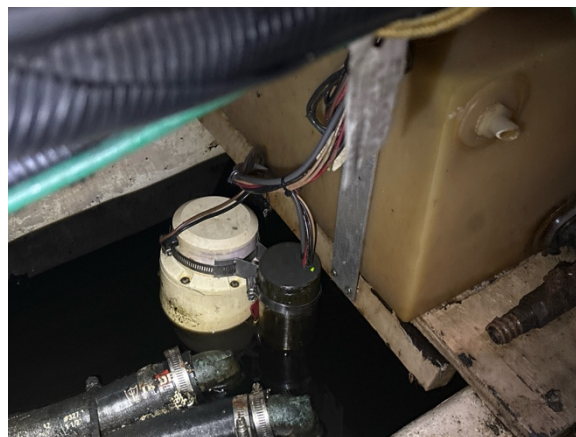
FWD engine room bilge pump
