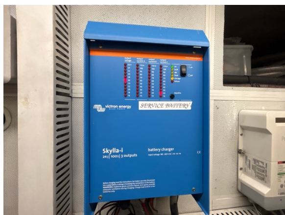
Service batteries charger
