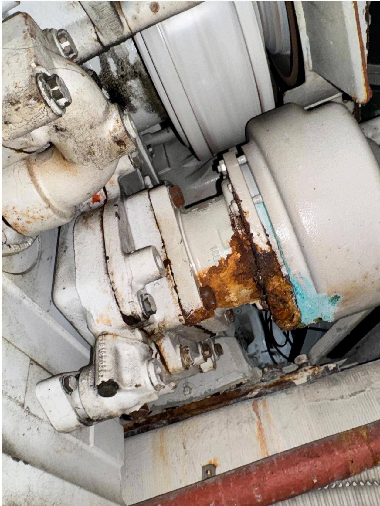
STARBOARD RAW WATER PUMP LEAK AND FRONT MAIN SEAL LEAK
