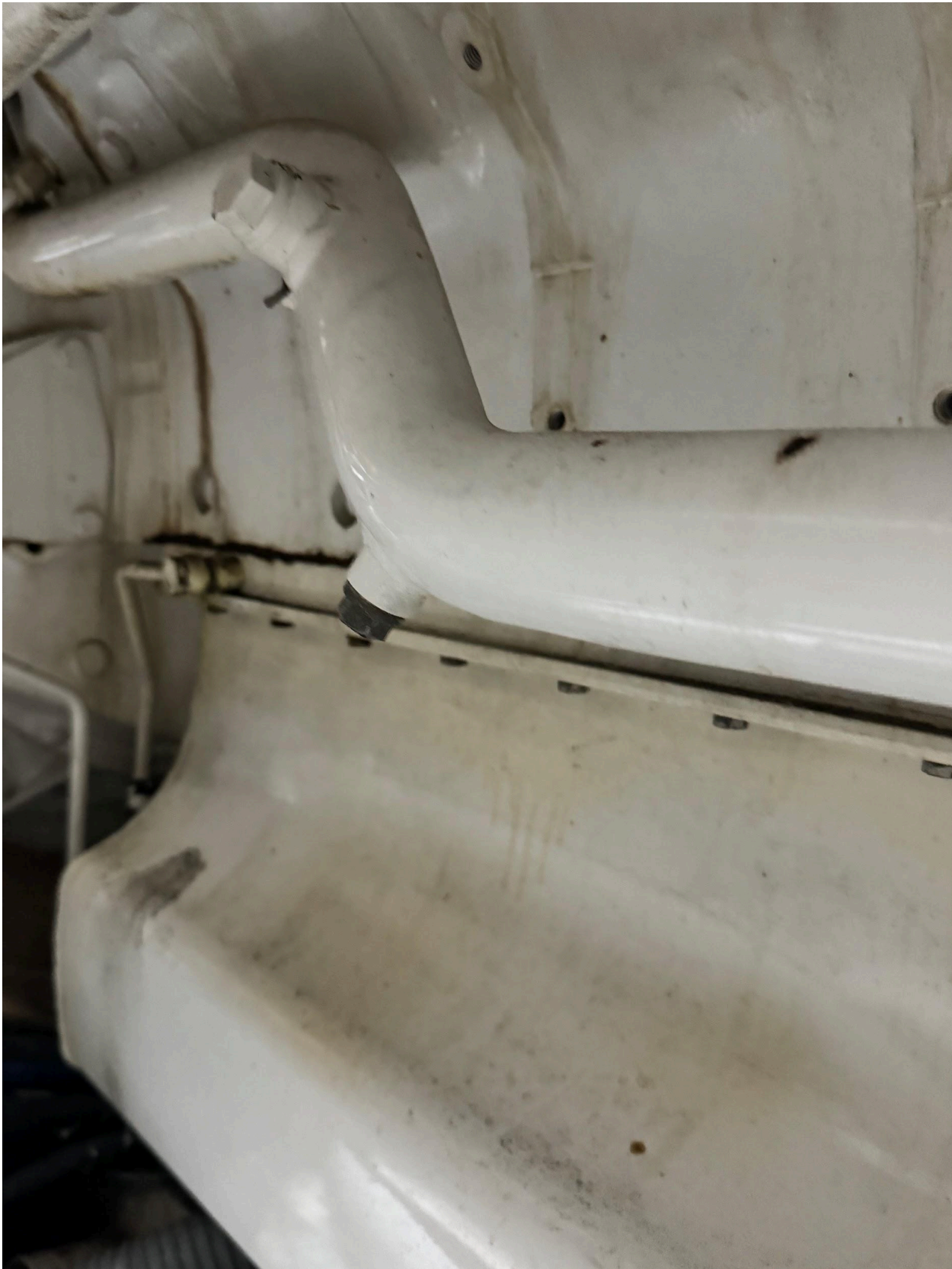
STARBOARD OIL PAN LEAK
