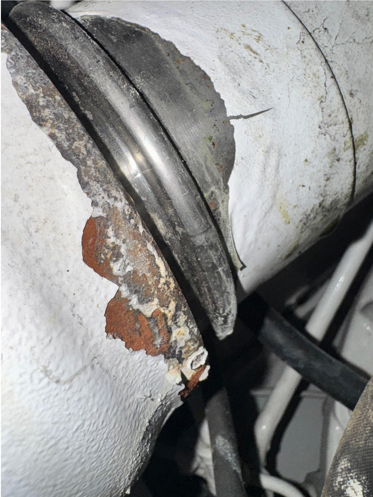
STARBOARD CROSSOVER PIPE COROSSION/ POSSIBLE LEAK
