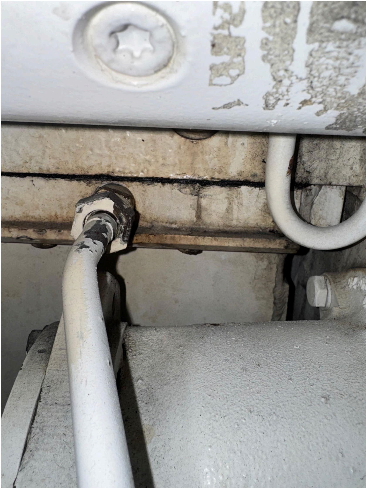
STARBOARD OIL PAN LEAK
