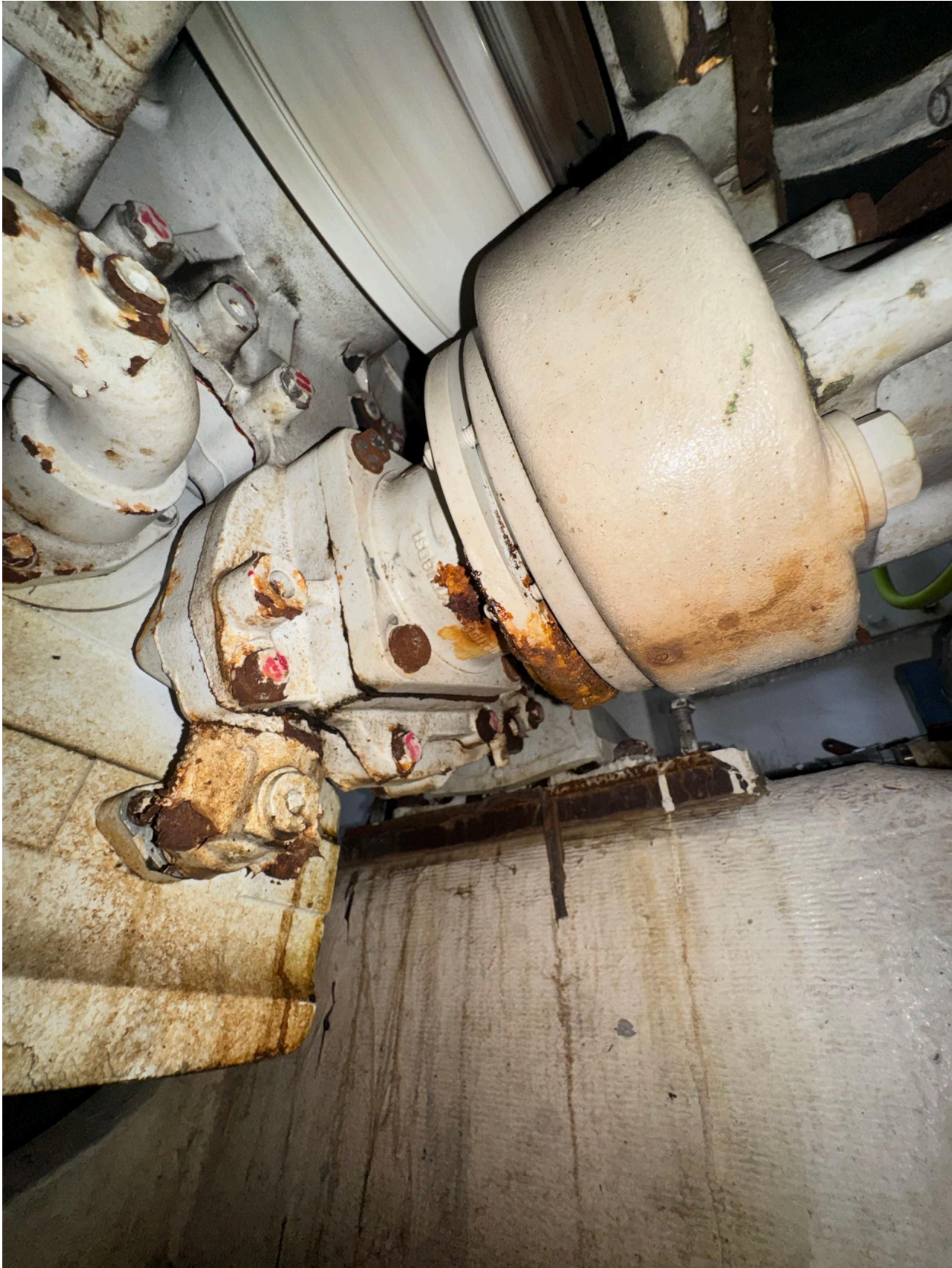
PORT RAW WATER PIMP LEAKING
