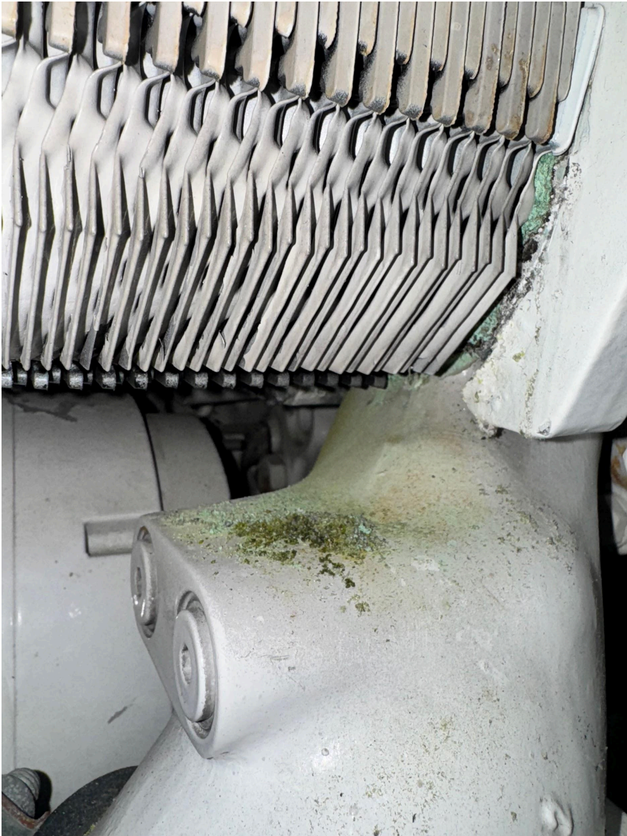
STARBOARD HEAT EXCHANGER RAW WATER PIPE
