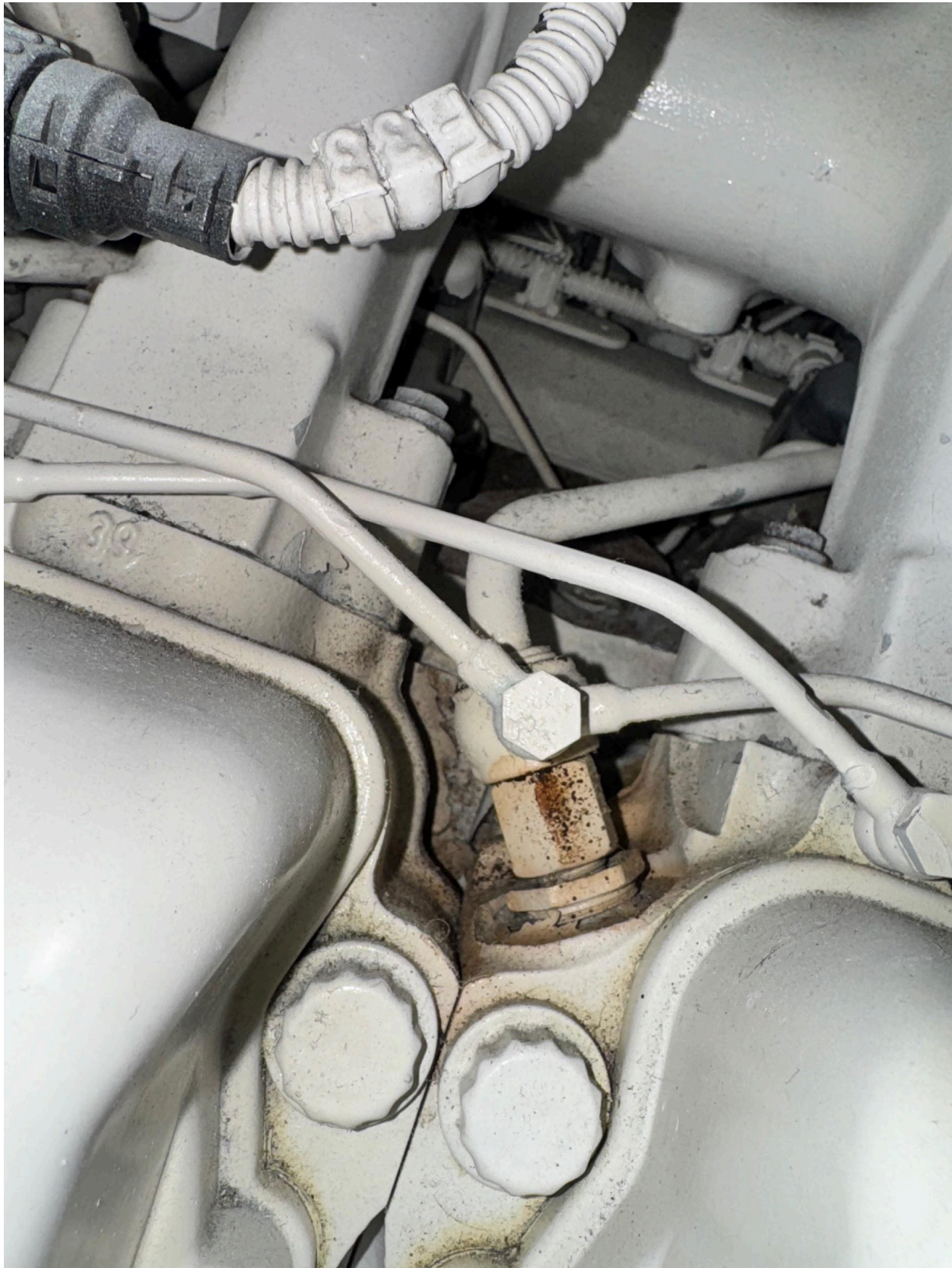
STARBOARD A7 HP FUEL LINE LEAK
