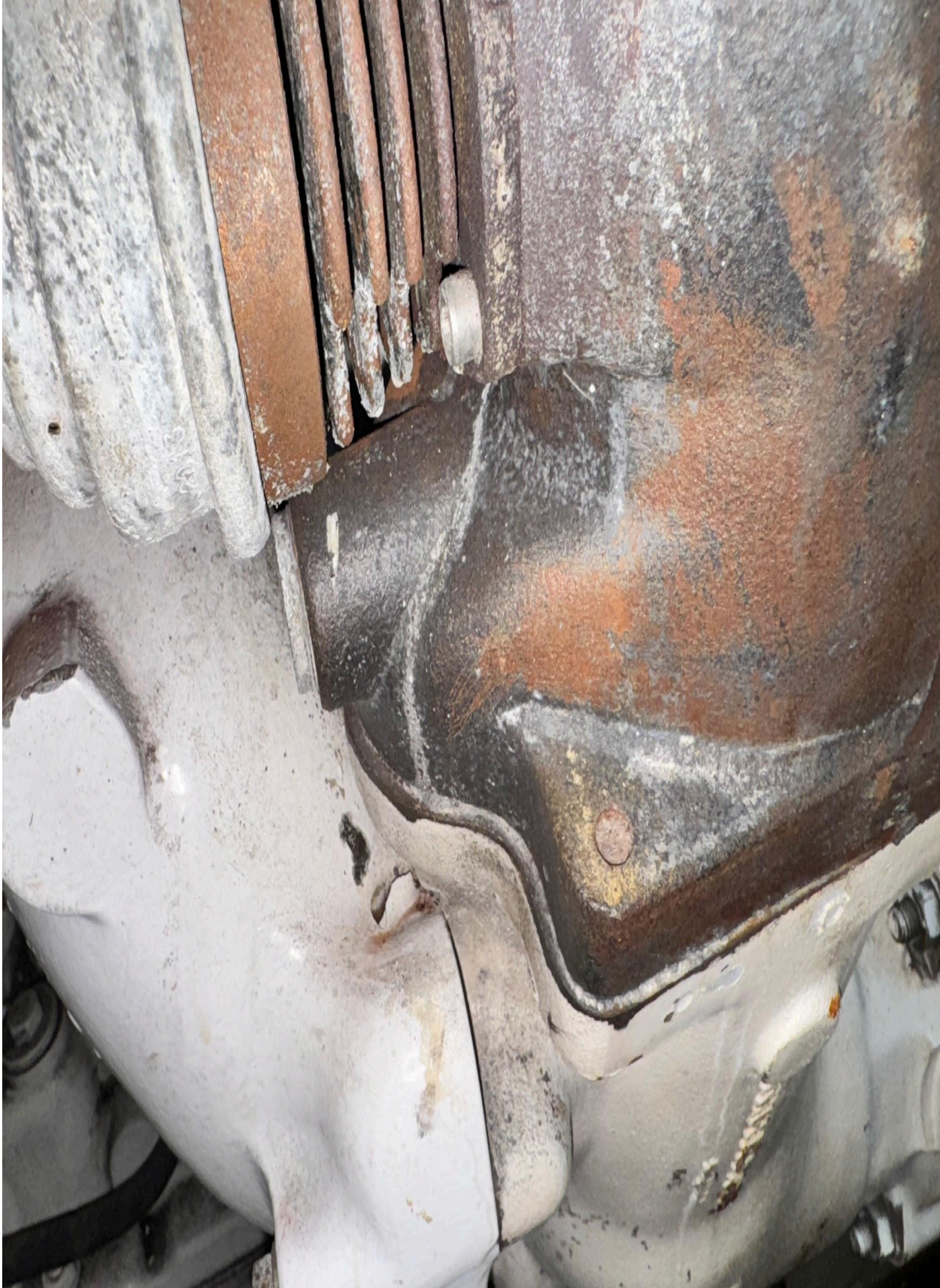
STARBOARD TURBO CORROSION AND START OF COOLANT LEAK
