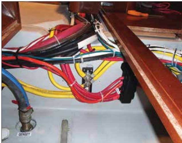
The modified battery well, seen here just before battery installation, had plenty of space to accommodate the new lithium models, as they occupied just half the footprint of the original AGM bank.
