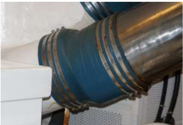
Figure 10.29 Stress on port hump hose
