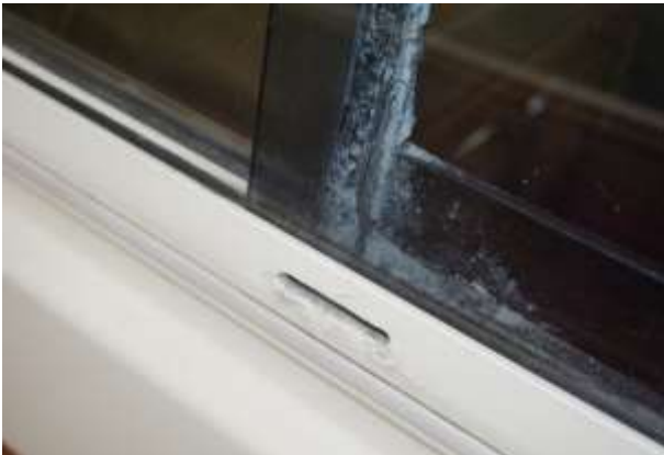
Figure 10.23 Corrosion on wheelhouse sliding windows
