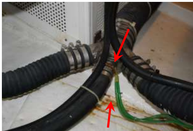
Figure 10.30 Stains indicate evidence of past/present leak on 3-way raw water diverter
