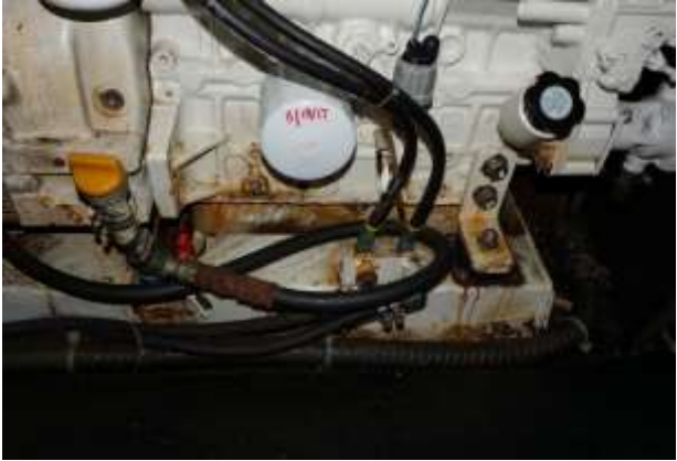
Figure 10.31 Corrosion on 16kw gen set
