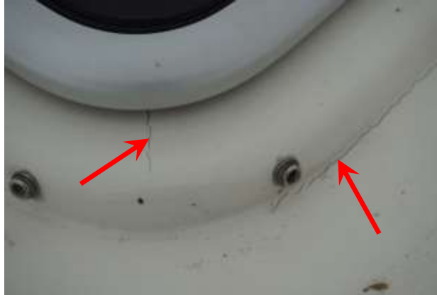
Figure 10.26 Cracks around deck hatch on top of wheelhouse
