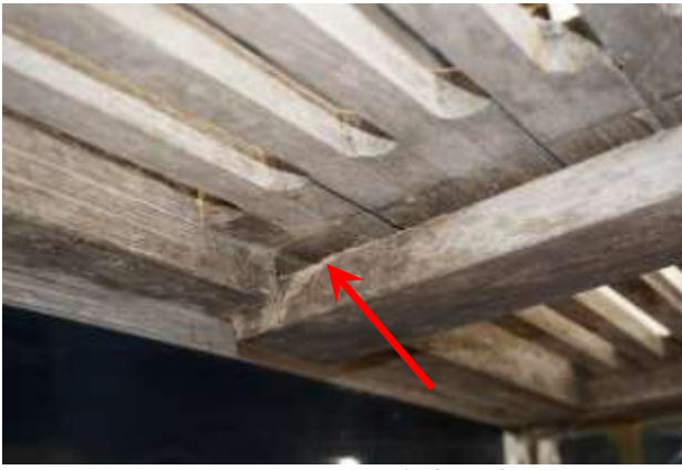
Figure 10.22 Loose swim platform framing
