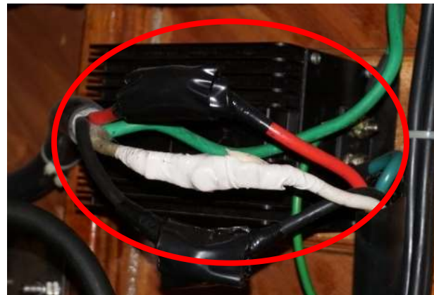
Figure 10.28 240-volt wire connections not in junction box
