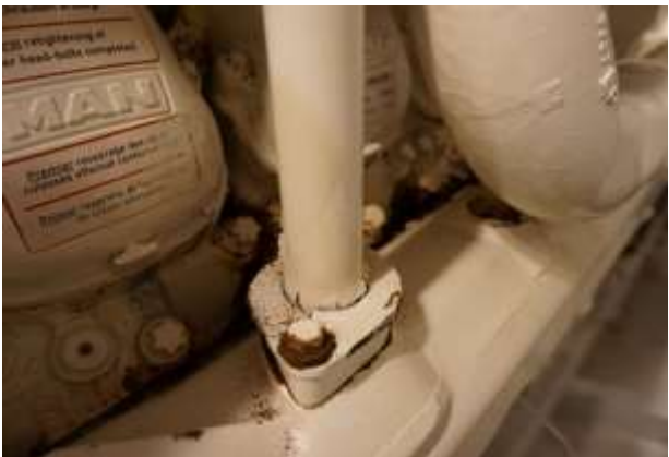
Figure 10.33 Surface corrosion beneath port engine intercooler thermostat
