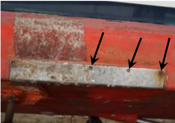
Figure 10.21 Missing & corroded fasteners on s.s. strap guards
