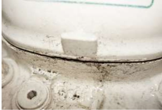
Figure 10.32 Small oil leak around port engine valve cover
