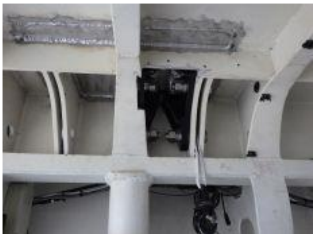
Chain plates from below deck
