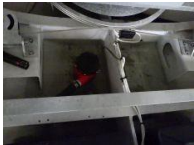
Bilge & pump fwd. of trim tab
