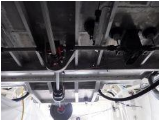
Grinder pedestal linkage from below
