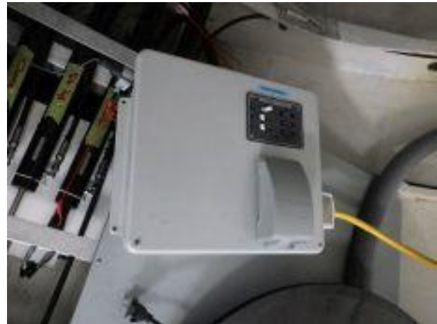
Shore power Junction box
