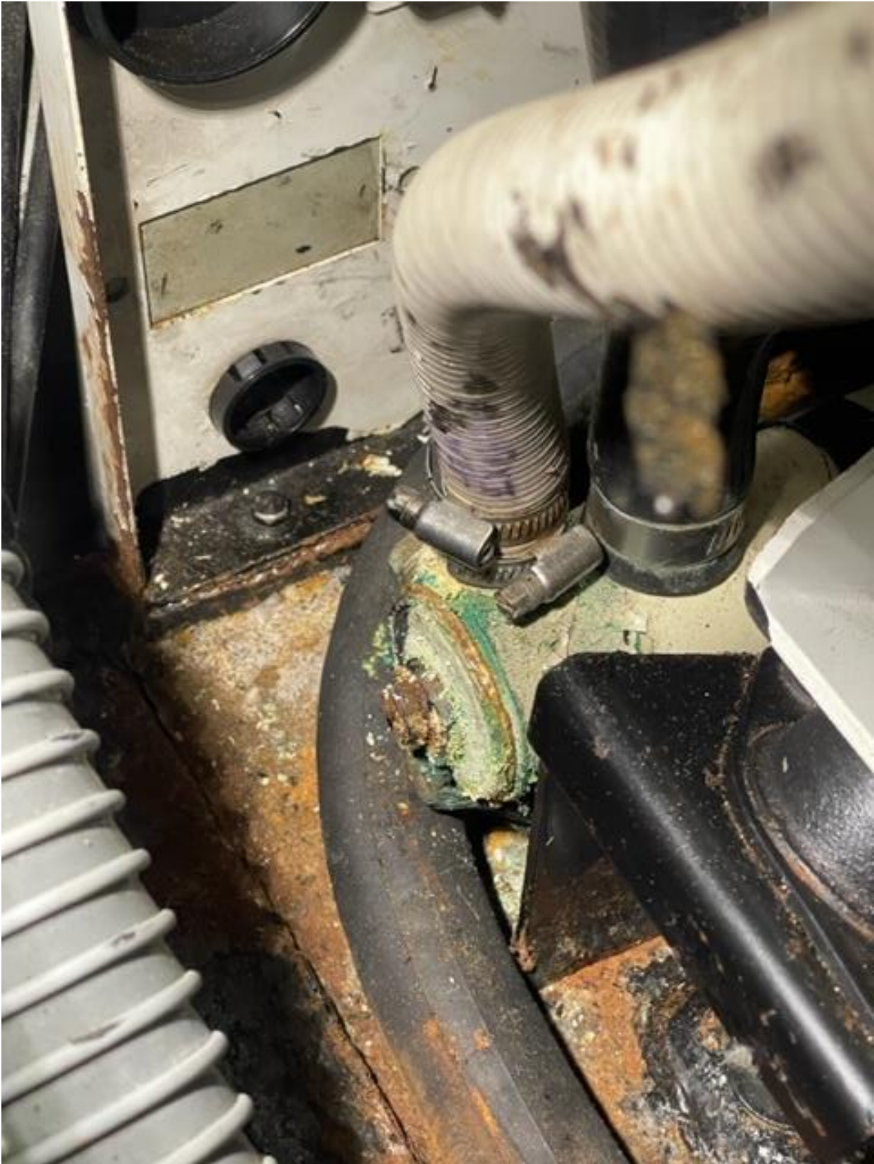
The generator heat exchanger end cap shows signs of corrosion. Recommended resealing it.
