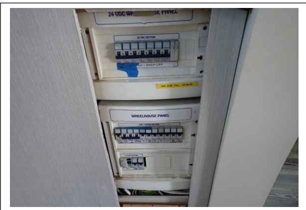
SUB ELECTRICAL PANEL
