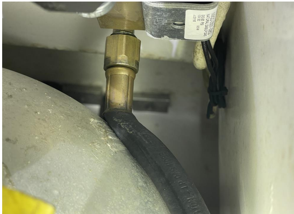
Below shows the kinked propane hose
