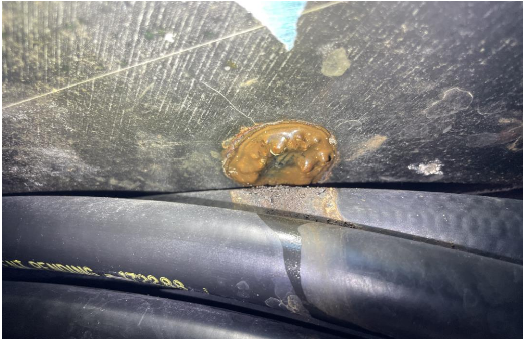
Above shows the weeping from the overhead centerline aft in the engine room
