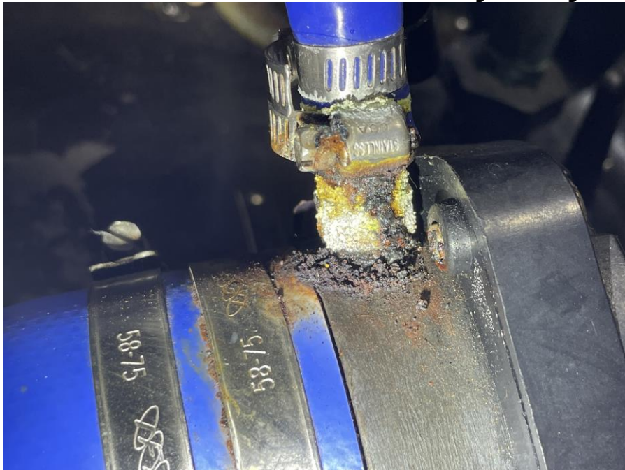
Below shows the corrosion at the shaft log cooling hose
