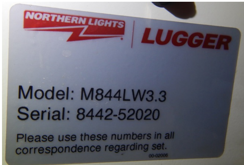
PORT Generator Label
