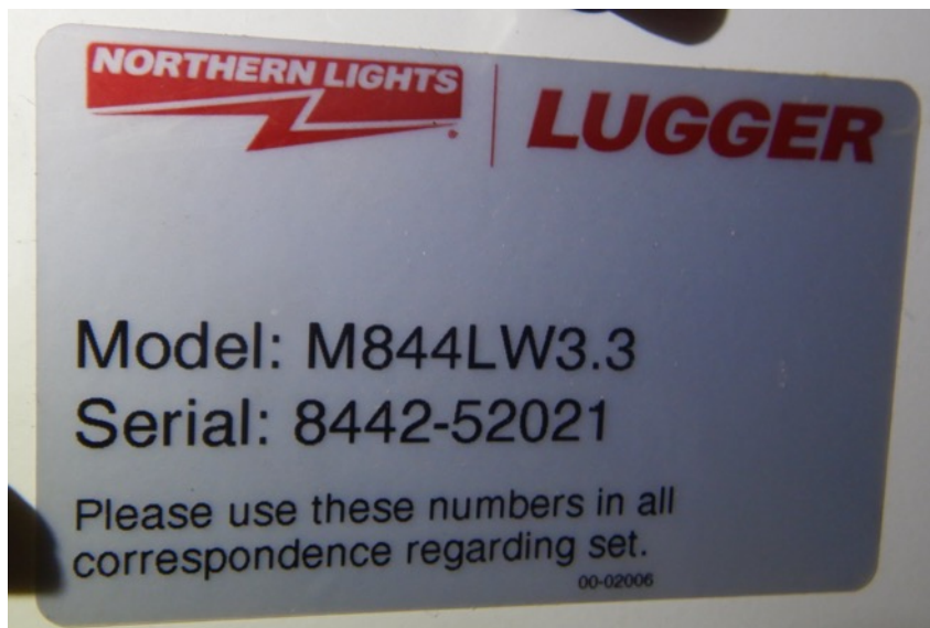
STBD Generator Label
